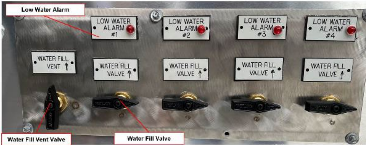
Water Fill Panel (Trailer Rear)
