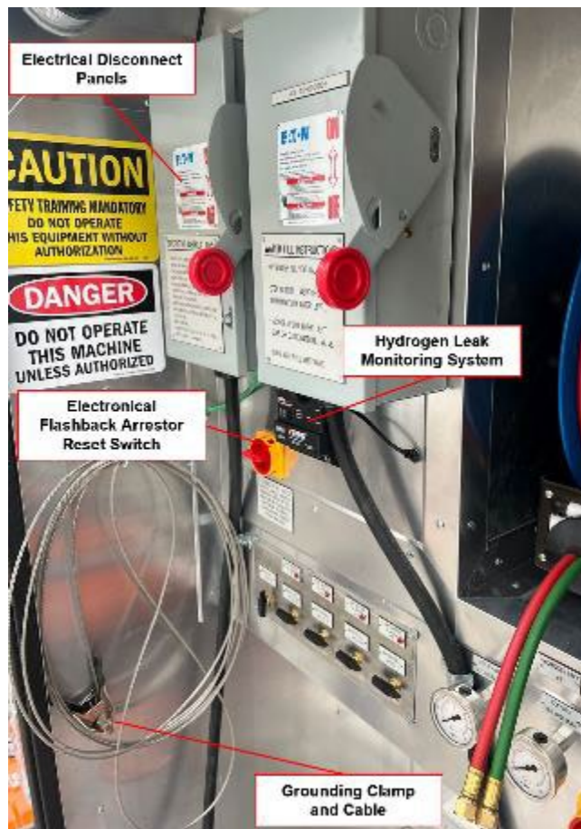
Electrical Disconnects and Safety Monitoring Systems (Trailer Rear)
